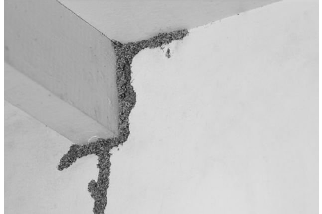
Example of termite mud tube.
